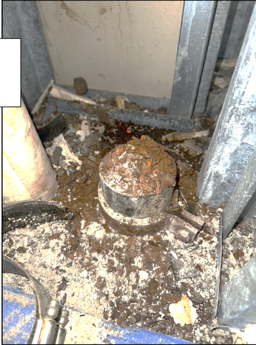
Impacted vent line with scaling debris
