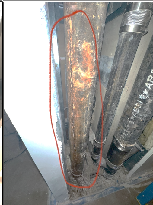
Cracked vent line in 01' stack
