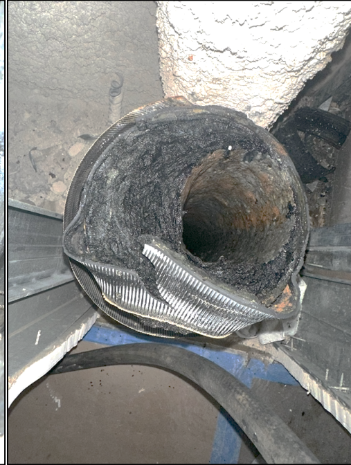
Impacted 6" main servicing 01' kitchen and clothes
