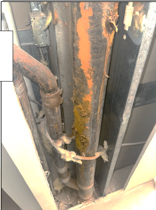
Exterior corrosion on 01' kitchen drain
