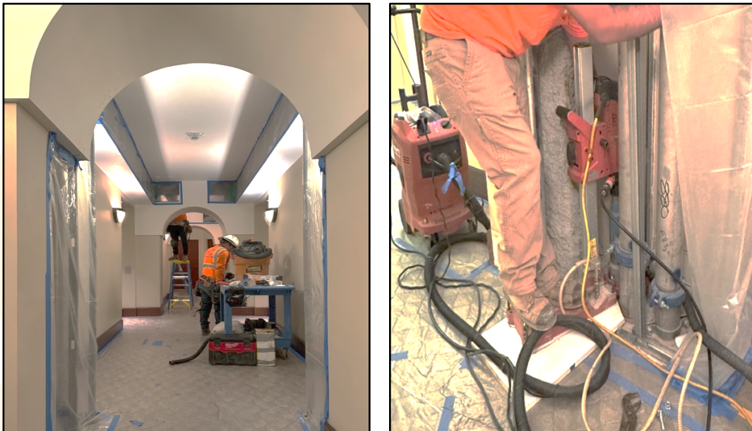
*Photos of distribution floor hallway preparation and active coring work for domestic routing.
