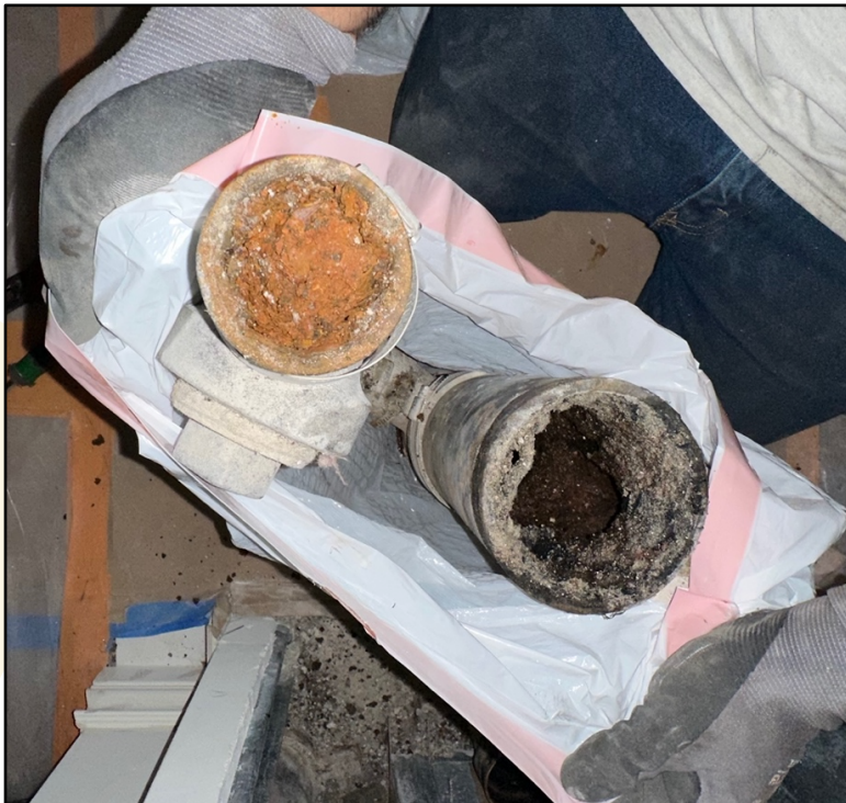
Impacted vent line in 03' stack
