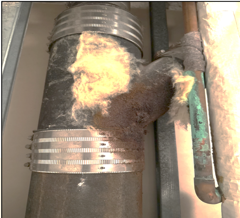
Corroded section of 6 inch main
