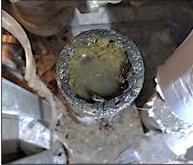
Impacted vent line in 03' stack
