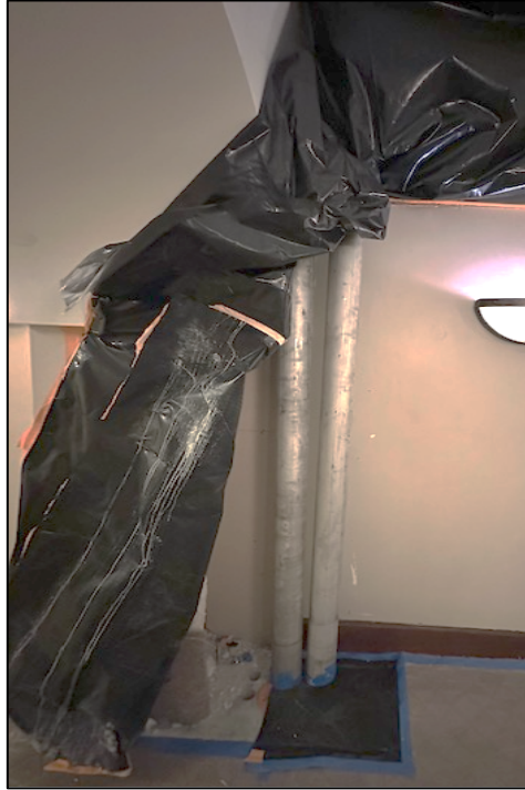
Common area domestic main on a common hallway
