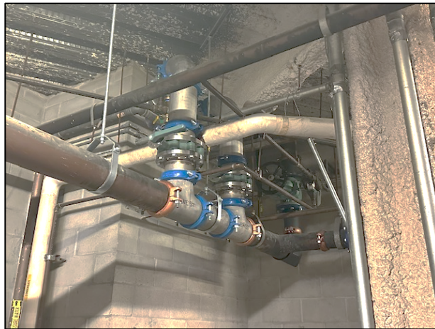
Domestic main connection in basement
